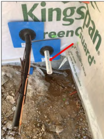
Sump pump discharge pipe
