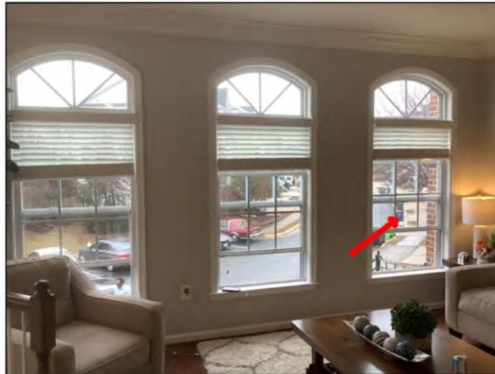
Difficult to operate
