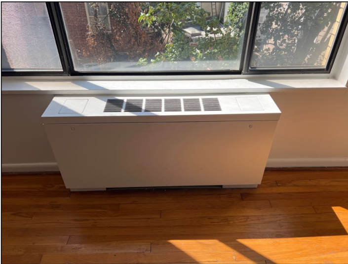
PTAC (fan coil)
