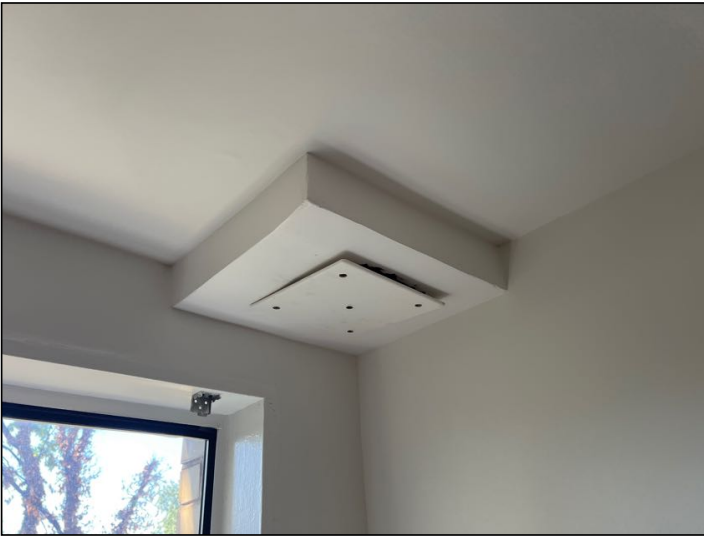
Loose access hatch
