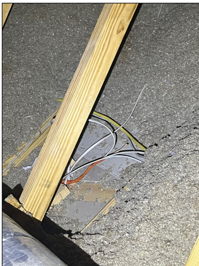
Missing insulation in some areas
