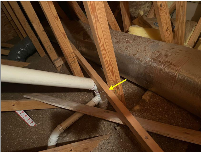
Loose bracing; Nails sticking outwards
