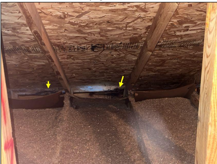
Stains and some deterioration noted to sheathing
