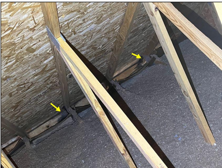
Signs of moisture intrusion
