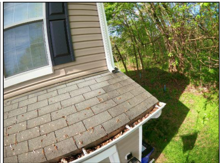
Terminates on roof, causing staining
