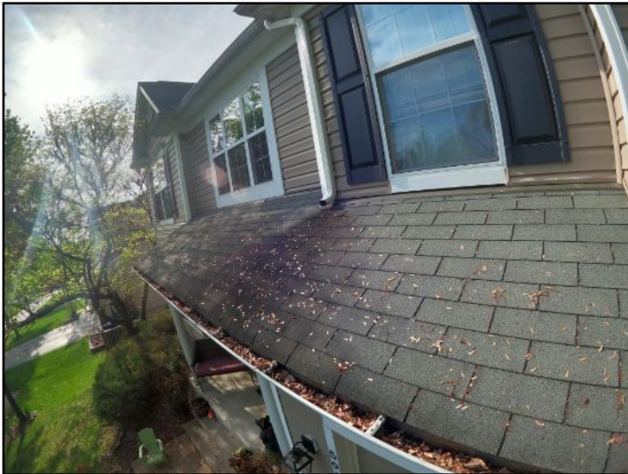
Terminates on roof, causing staining
