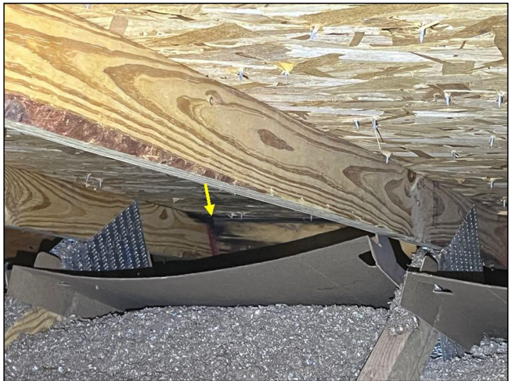
Signs of moisture intrusion
